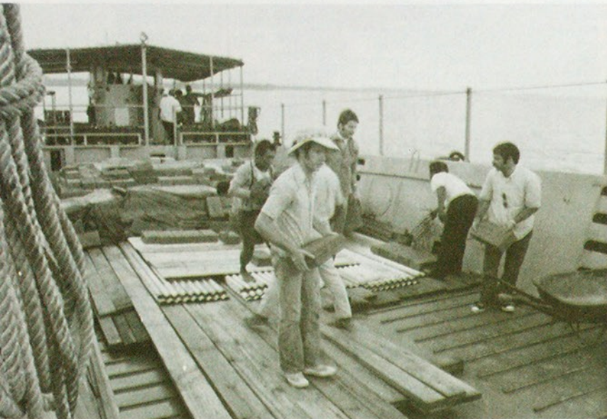
During January, nine students from Evangel College went to Panama to build a church on the tiny tropical island of Isla Tigre. The students were transported to the island along with five tons of construction materials, by the U.S. Army Forces Southern Command in one of their landing craft (LCM). Calvin LeMon, director of campus ministries (right), went with the students.
