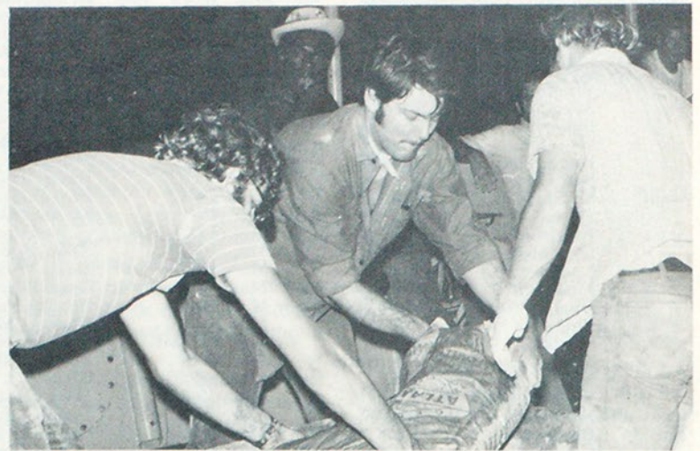
Students began unloading the building materials, including cement and blocks, upon their arrival on Isla Tigre. To meet their goal of building the church in five days, the students had to lay 400 cement blocks a day under blistering tropical sun.
