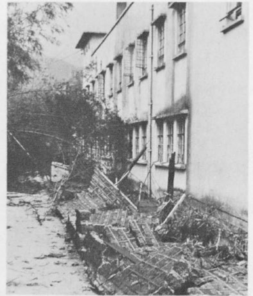
The granite stone wall was wrecked by the force of the tidal wave.
