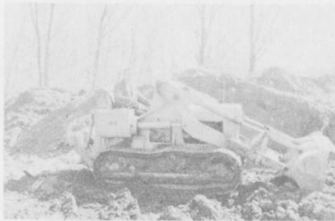
Bulldozer breaks ground for the new Assemblies of God church in Norwalk.
