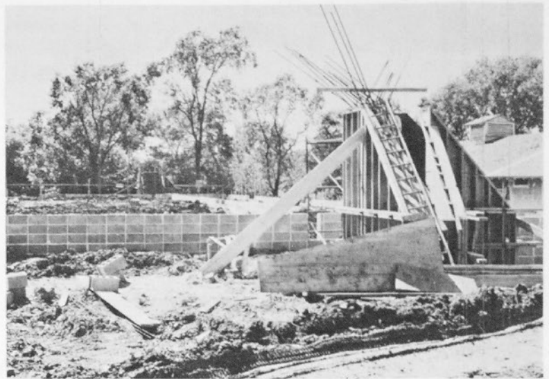
The activities building, under construction at Evangel College, will contain a regulation basketball court with bleachers for 1,500, other physical education facilities, and faculty offices.
