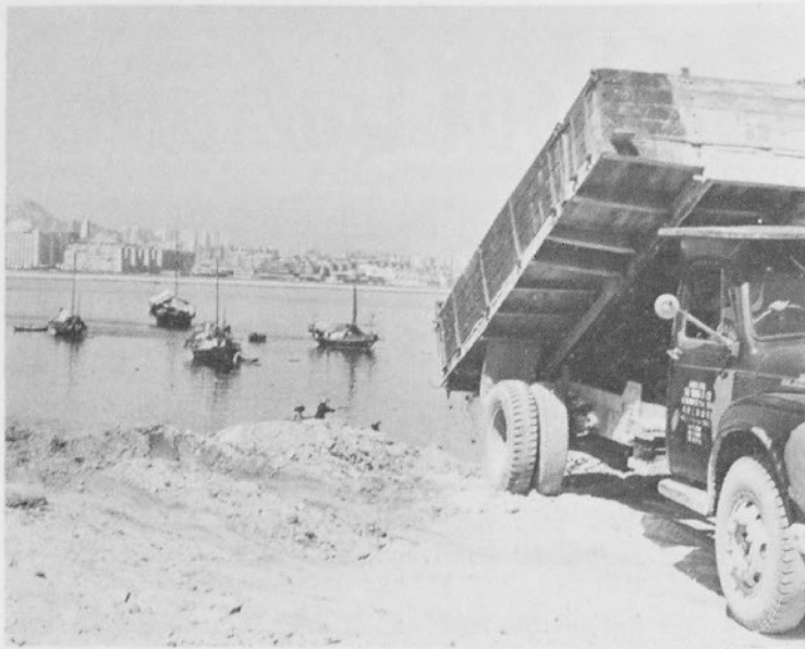
Hong Kong work crews level mountains and fill in the ocean to make room for people to live.
