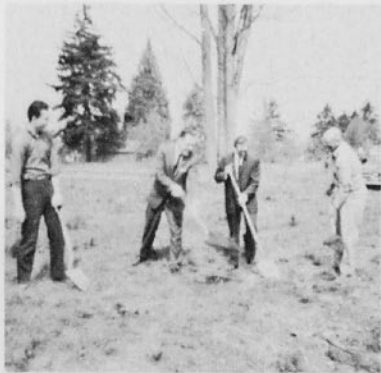
Ground breaking for new food service building on NBC campus was a joyous occasion. Left to right: Lowell Wood, John W. Lackey, B. P. Birkeland, and H. J. Secrist.
