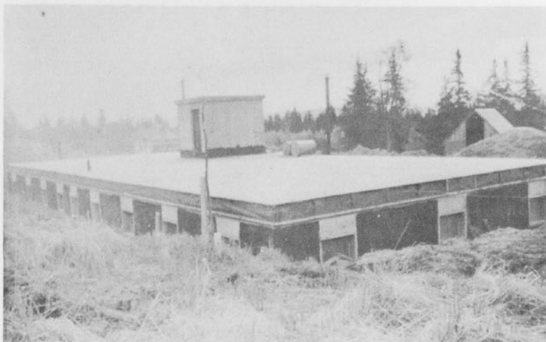
Services are held in the completed basement of the new church being erected at Homer, Alaska.
