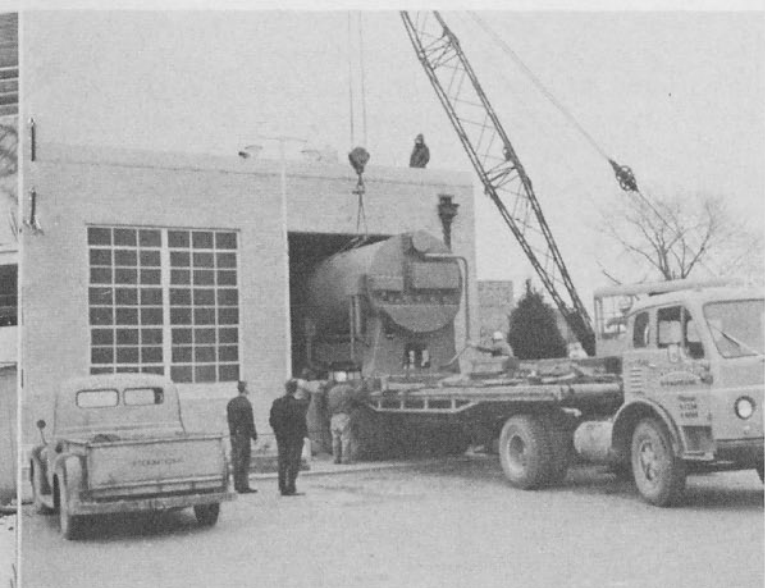
Additional 400-ton capacity air conditioner unit was moved into power plant to serve the new building.
