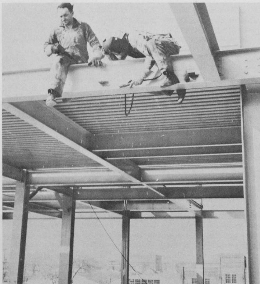
In freezing weather, welders worked on top floor installing brackets to hold aluminum frames for curtain wall.
