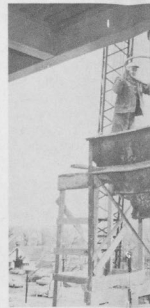
A 100-foot boom crane hoisted concrete to hopper on top of building.
