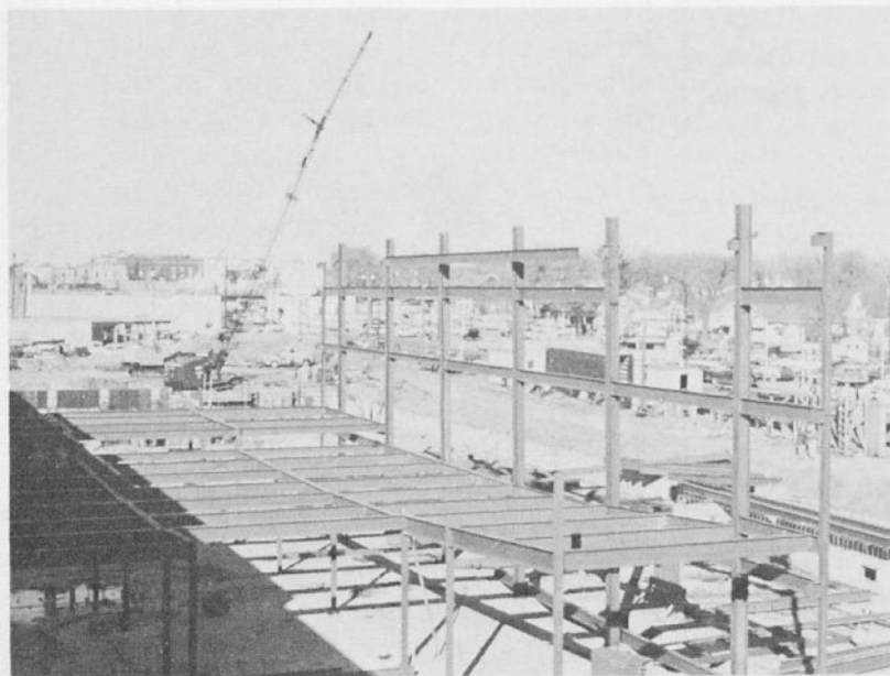
The first section to rise above the ground floor was the chapel. The floor slopes down from the foreground toward the raised platform at the far end.
