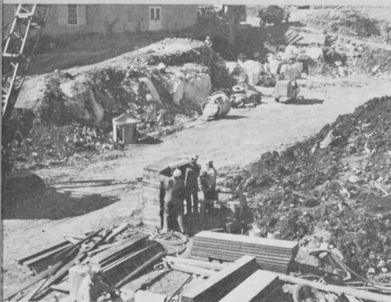
Ground was broken on August 2. A month later most of the excavating had been done but work was slowed by the unexpectedly large amount of solid limestone to be blasted.
