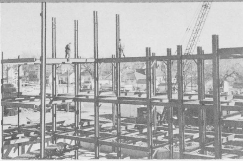
Up on the level of the fourth floor, these men could get a good view of the job but they did not dare to glance about them as they walked along the narrow I-beams.
