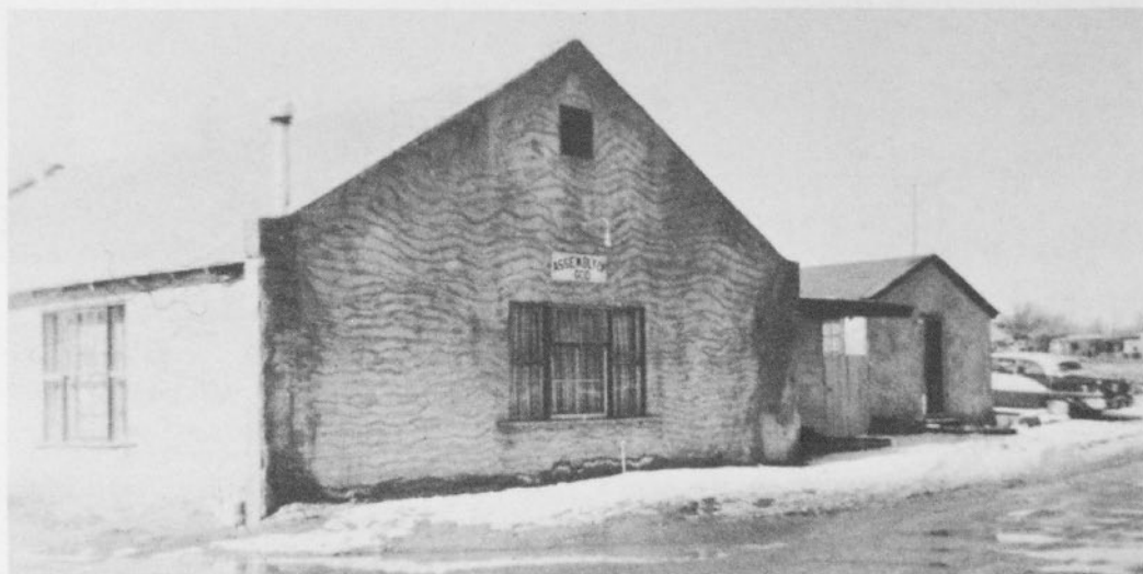
The church and parsonage both need new stucco and paint
