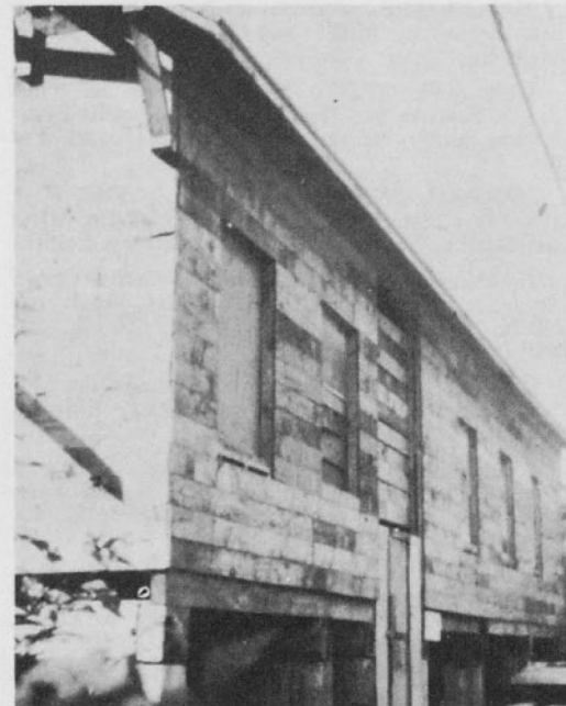
The unfinished exterior of the church building at Sitka, only partially rebuilt since fire broke out in 1954. Costly materials are needed to enclose it for cold weather use.
