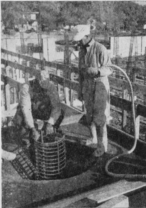
Workmen prepare to lower the strange jogging machine down into a pillar form to settle and jog down the concrete which is going into the form to make the pillar. Notice the circular reinforcing steel.
