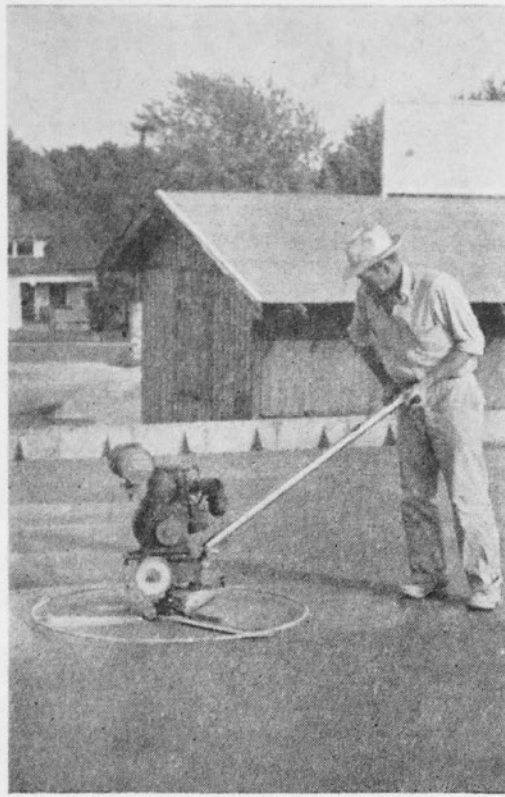
The cement-smoothing machine simply whirls its blades around at high speed, giving a smooth and level surface to the newly-poured concrete floor on which the big printing presses will be placed.
