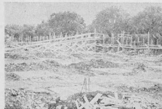
Special runways had to be built on which to carry the concrete to the proper places along the wall forms.
