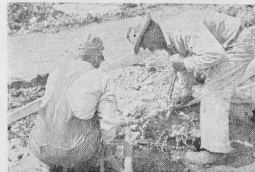
Plumbers were brought in to rig up special lines to provide water which is needed in the mixing of concrete.
