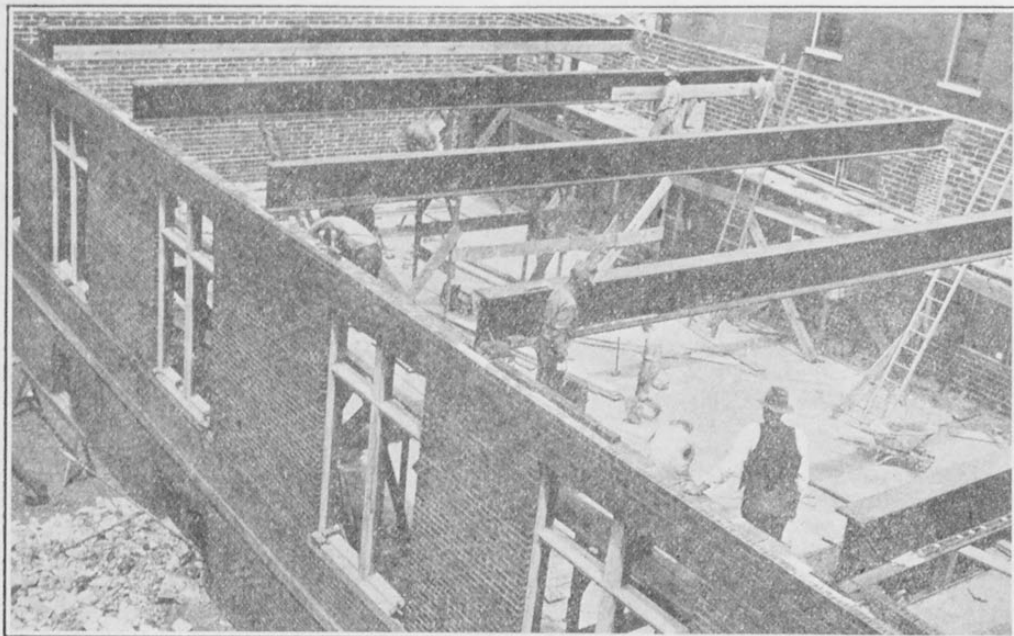
Work in progress in new addition to Central Bible Institute. Can you see your bricks? Plenty more needed. Read article below.
