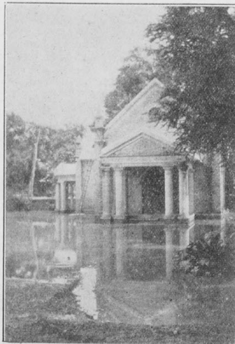
Chapel damaged by flood, Chapra, India. Foundation and steps under water.
