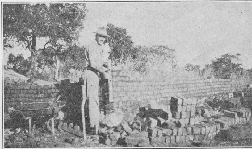
Building for God in Africa. John Richards at work at their new mission station
