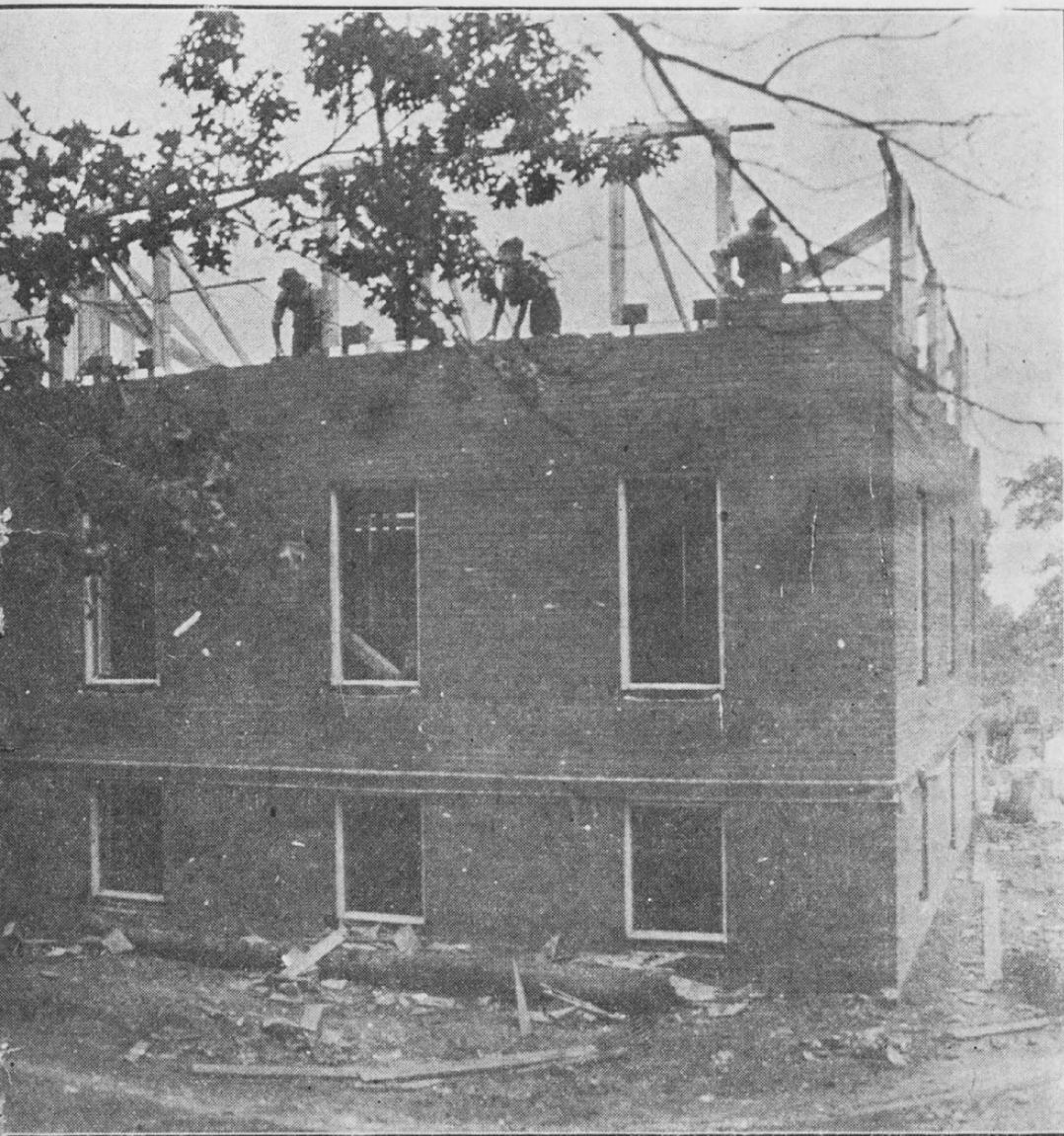
this picture was taken they are about up to the top of the second story. The picture shows the money paid for up to date, but funds are needed to push the work to completion.
