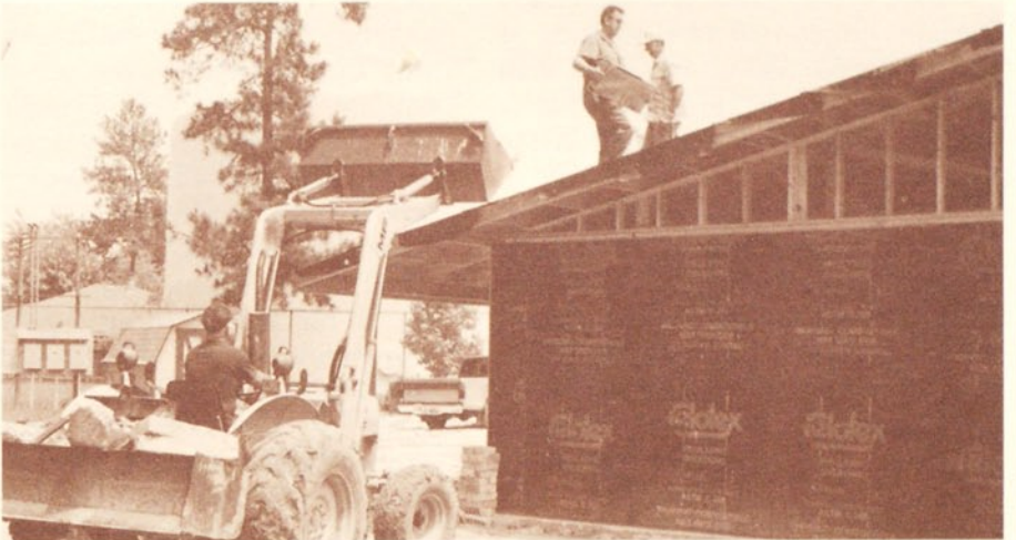
It takes many skills to make a project run smoothly. Here a tractor operator supplies roofing materials the easy way while the men on the roof nail on the shingles.
