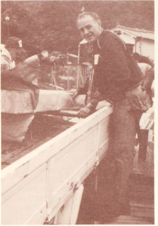
DHM MAPS Department Secretary Patrick Donadio pitches in on this building project, helping to unload laminated beams.
